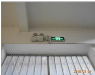
Photo of fire safety equipment Emergency light and Exit sign.JPG
